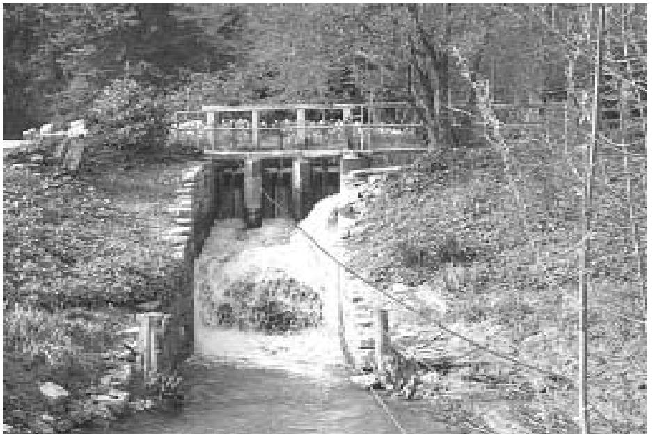
Water rushes through the new stonework and oak structures that make up the new working sluice.
